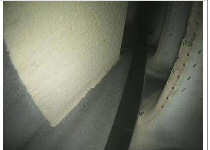
HPTN1 T/E Inner Platform.
