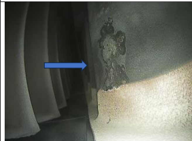
HPTN2 T/E and Outer Platform. Note erosion/deposits?
