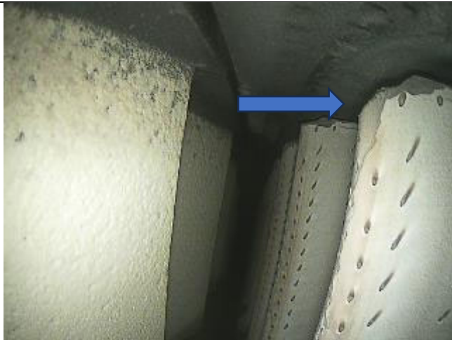
HPTN1 T/E Outer Platform. Note tip damage.
